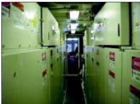
Well lit center aisle of the ALP-46.
